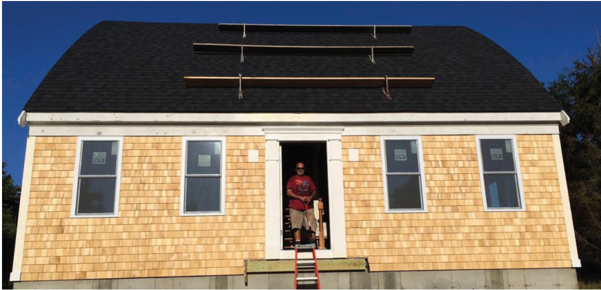
New affordable housing under construction in Nantucket. (Photo provided by Housing Nantucket.)
